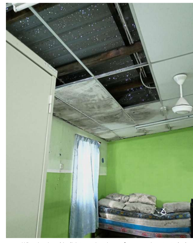
▲ When it rains, this disintegrating zinc roof causes rainwater to leak through the ceiling panels, flooding the boys' dormitory at Rumah Titian Kaseh Asrama Putera in Taman Duta, Kuala Lumpur.
